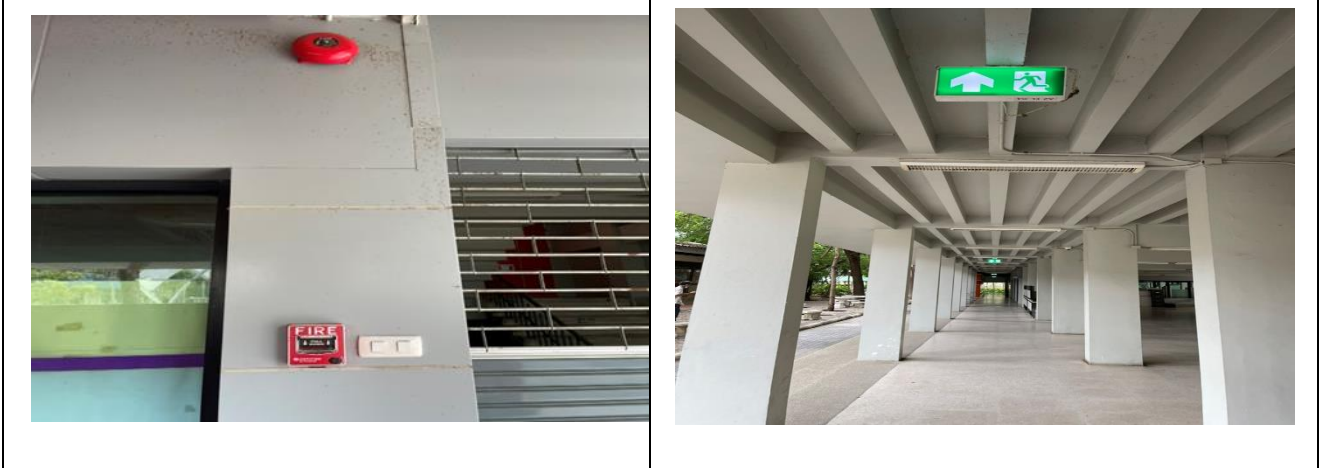
Fire Alarm System
