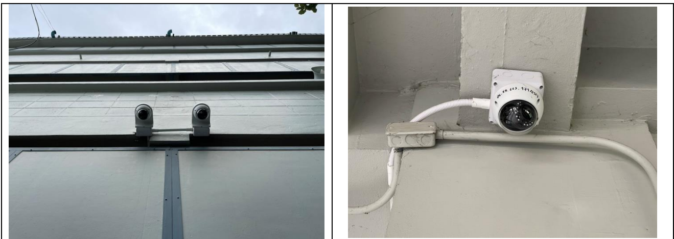
Example of CCTV in and out of the buildings around the campus
